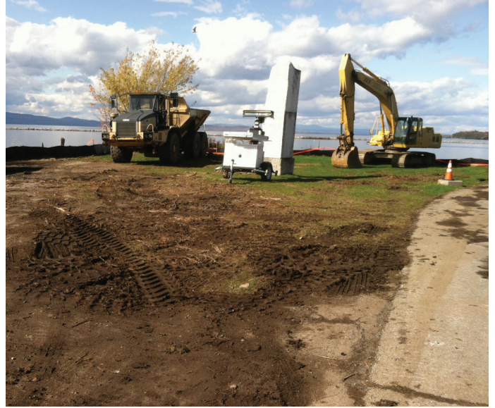
Pause place rehabilitation work between Roundhouse Park and Perkins Pier along the Path
